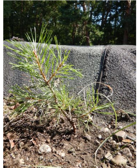
Dak [3]: plantengroei in/tussen roofing.
